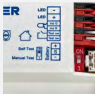
Self test & manual test switch
